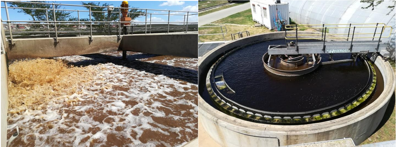
Figure 2.3: Activated sludge aeration basin (left) and clarifier (right) used to treat brewery effluent.
